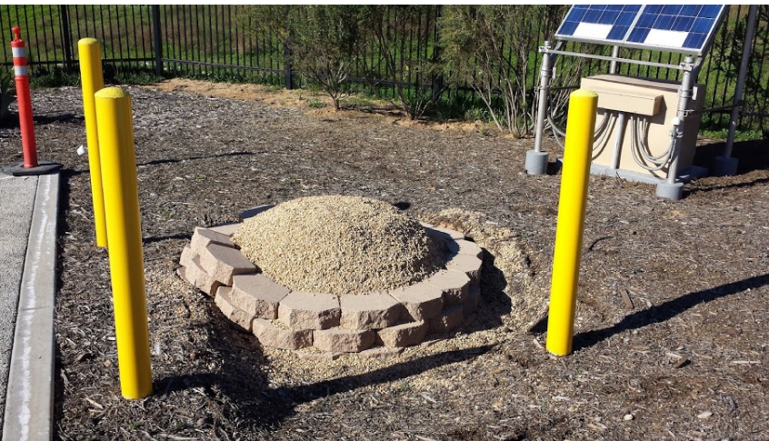
Figure 3. Subsidence at EOCG. Note the seismic vault has clearly subsided, and the yellow posts have been recently installed. Photo courtesy of Dan Determan, USGS. Photo taken on January 6, 2015.
