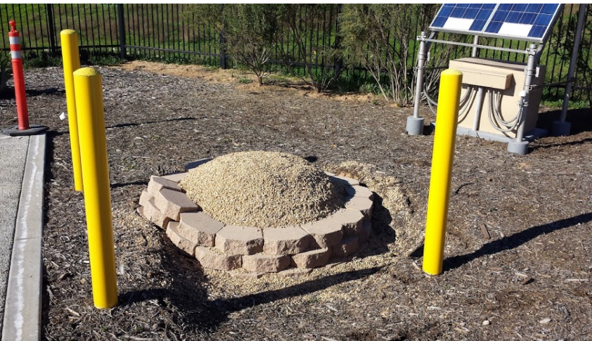
Figure 3. Subsidence at EOCG. Note the seismic vault has clearly subsided, and the yellow posts have been recently installed. Photo courtesy of Dan Determan, USGS. Photo taken on January 6, 2015.
